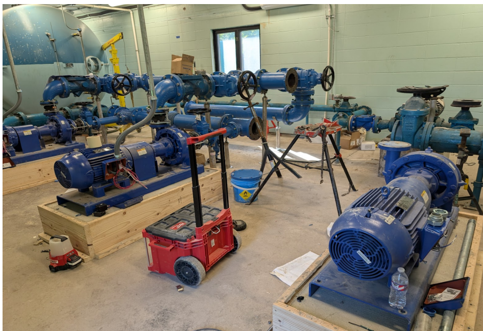
Lum Booster Station New Booster Pumps
